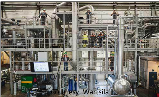
CO2 capture test facility at Wartsila Moss
