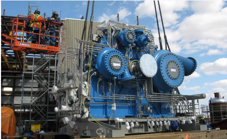
Figure 4: MAN Energy Solutions is installing three compressors at a large-scale carbon capture project in the port area of Rotterdam, Netherlands. It is planned to store approximately 2.5 million tons of CO 2 per year under the North Sea
